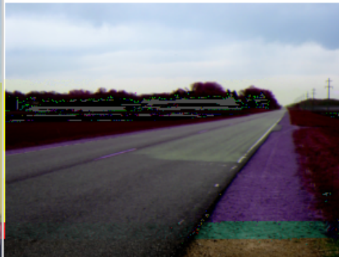
MN 251 Showing 4-Yr Old Fogged Section (back) Repelling Moisture during Light Rain Storm While Water is Penetrating into Unfogged Section (foreground)
